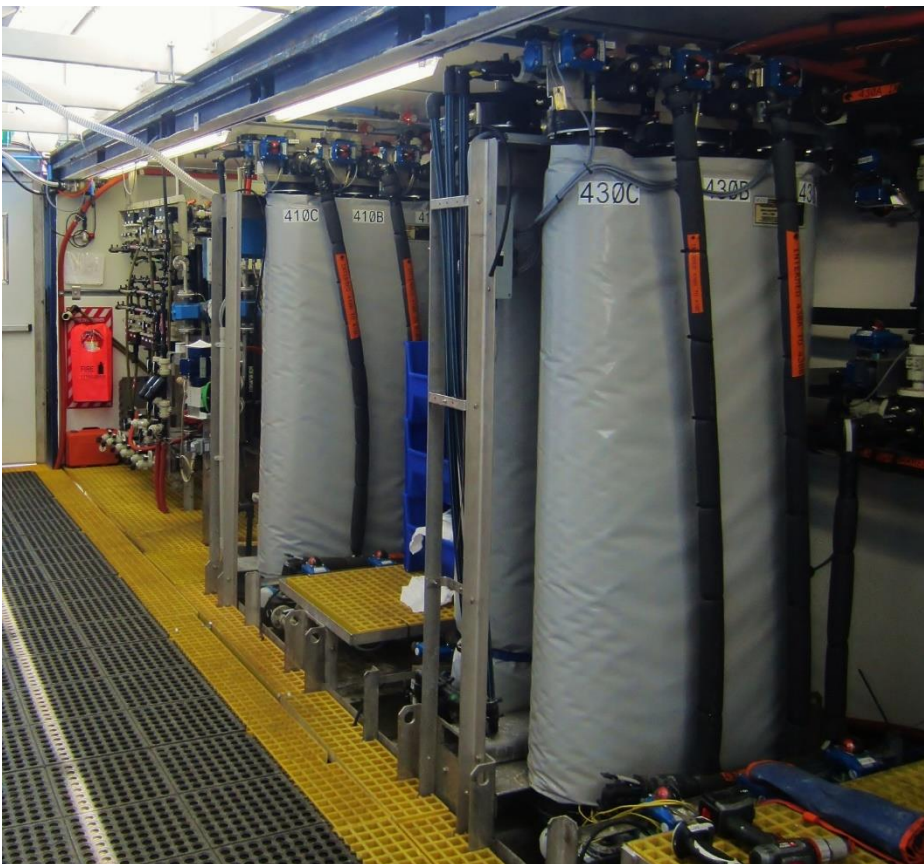
Extraction vessels in the Demonstration Plant
